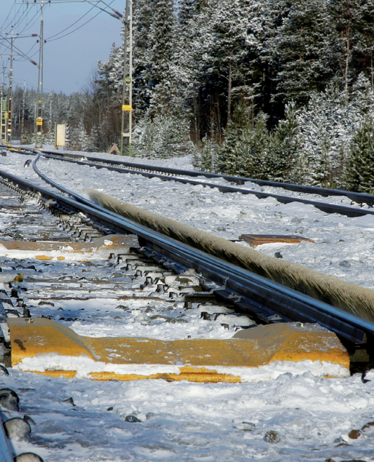
Brush and heater creates the snow free zone.
